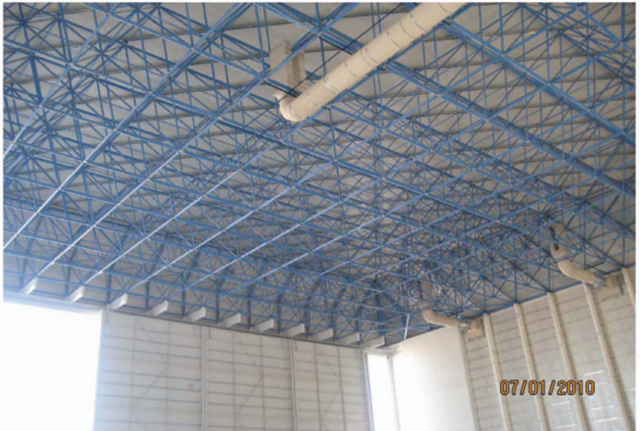
Figure 11. Inside view of the completed airbus a380 aircraft hangar and large doors
