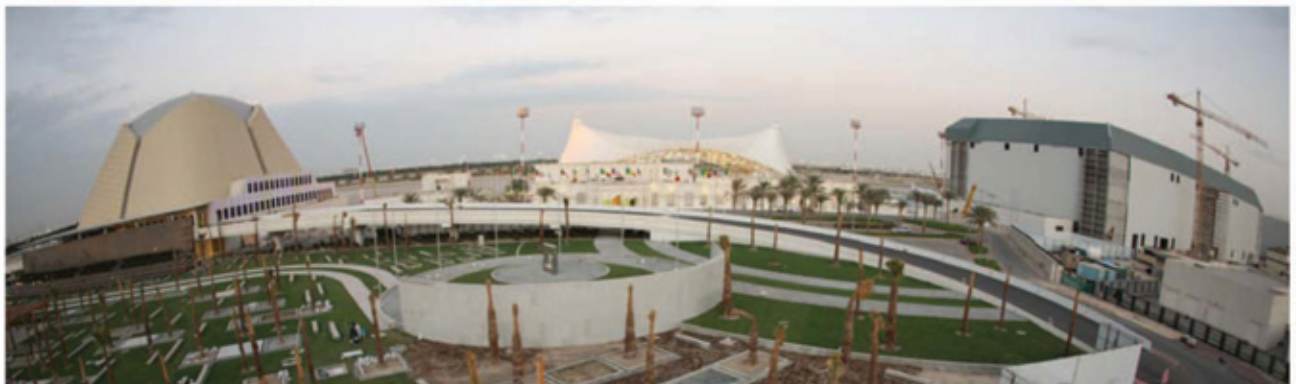
Figure 21. General outside view of the space frames constructed in Kuwait International Airport
